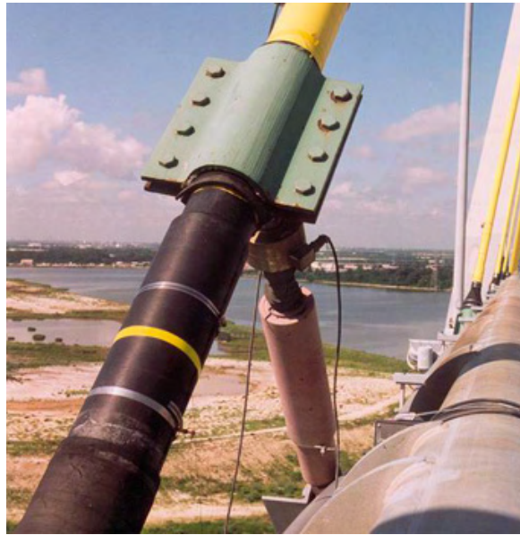
Figure 6.6 Type I WDP damper installed on stay AS16
