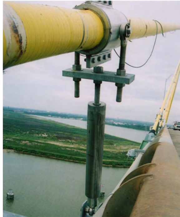
Figure 6.20 Type II WDP damper installed on stay AS24
