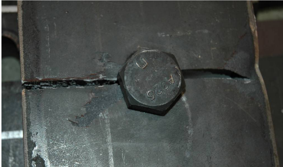
Figure 4.58 Typical Crack Orientation for Thick Plates ( \geq 1.0 Inches) with a Gusset Plate (Specimen E-3)
