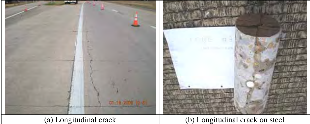
Figure 4.9: Longitudinal cracking on steel
