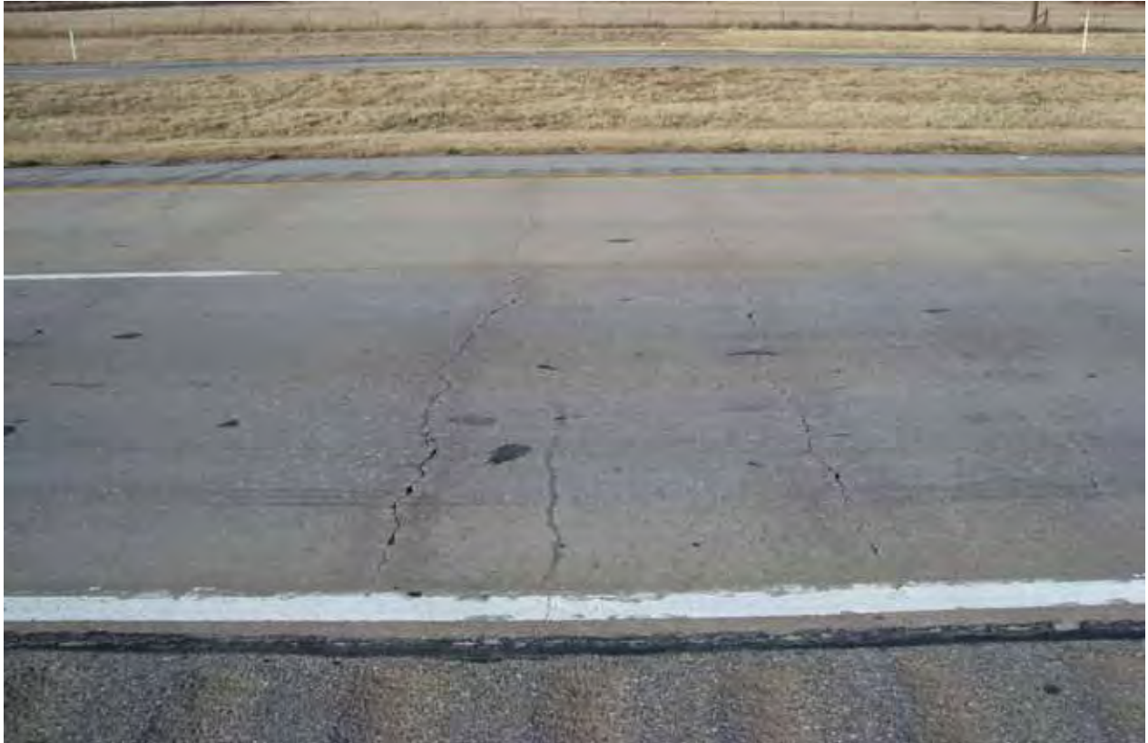
Figure 4.11: Transverse fatigue crack formed between two old transverse cracks
