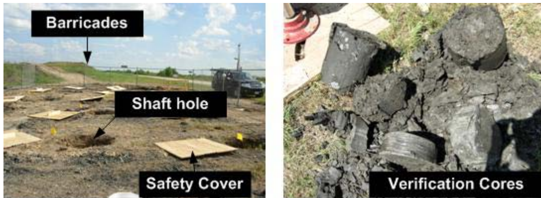
Figure 1.6.7 Site landscape after finishing drilling 18 non-production shaft holes (left) and the verification cores obtained (right)
