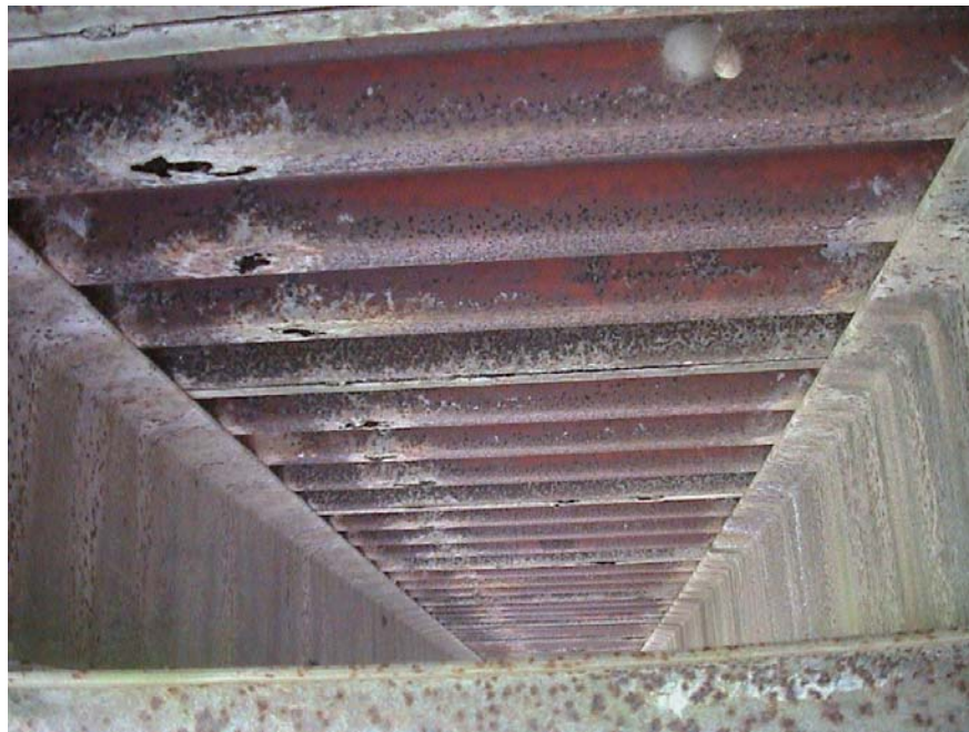
Figure 1.3 Corrosion in Bridge Deck
