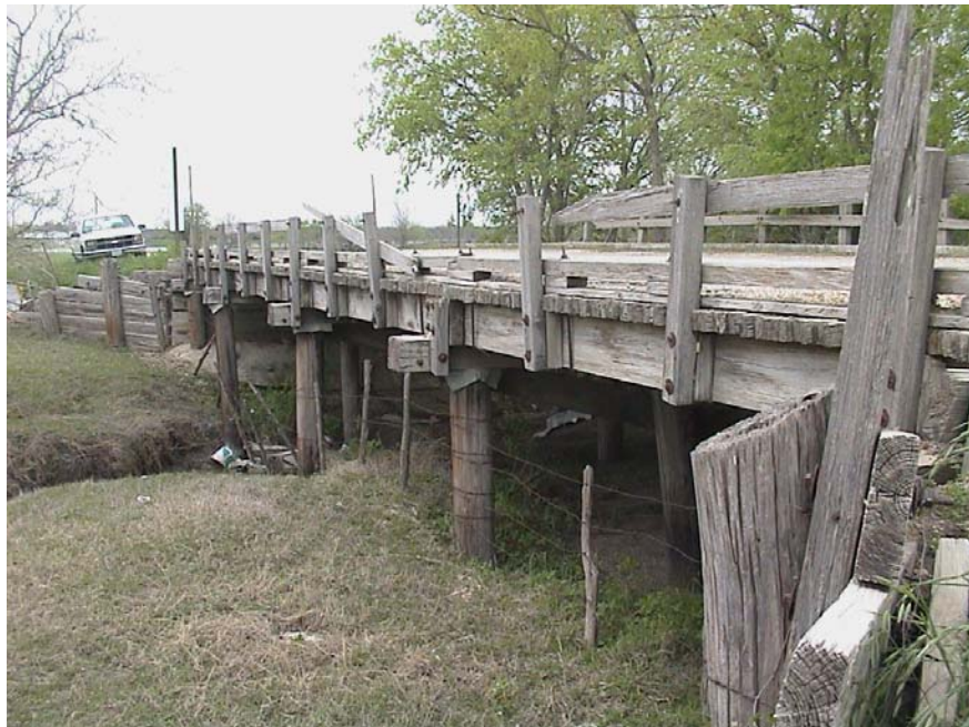
Figure 1.7 Broken Wooden Guard Rail
