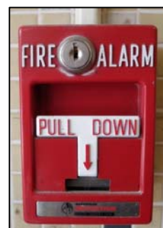
Fire alarm pull station
