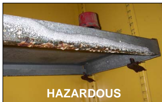
Rusted shelf supports
