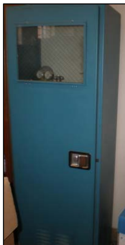
Compressed gas cylinder cabinet
