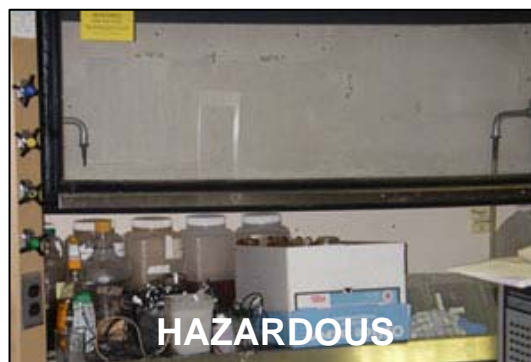
Improper storage in a fume hood
