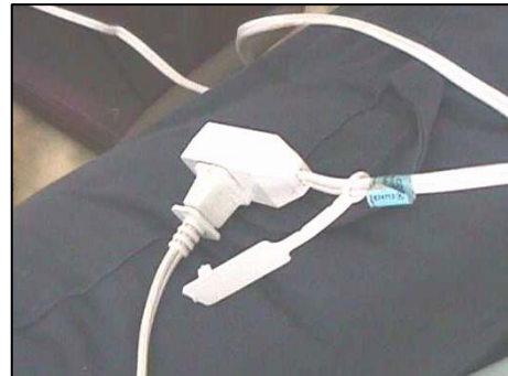
Electrical cords daisy-chained
