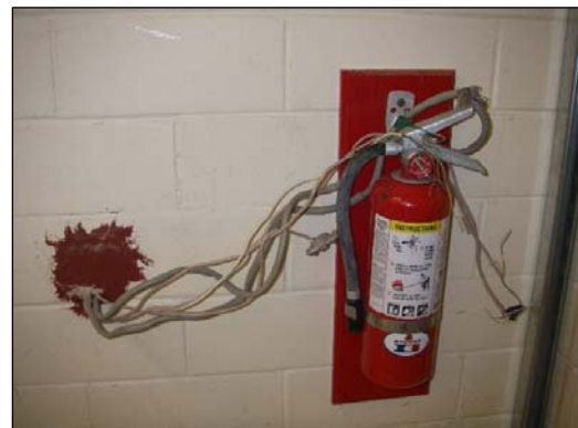
Blocked fire extinguisher
