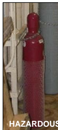
Unacceptable method of securing a gas cylinder
