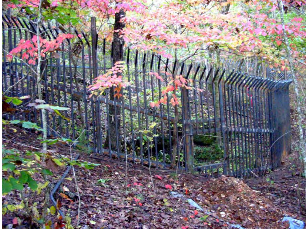
A 10-foot-high, vertical bar fence around a pit entrance in Missouri. The access door is temporarily open. By Jim Kaufmann and Kenny Sherrill.
